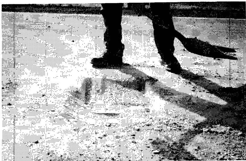
Figure 7. a. Recommended orientation of milled patch, b. Milled patch with rounded edges
